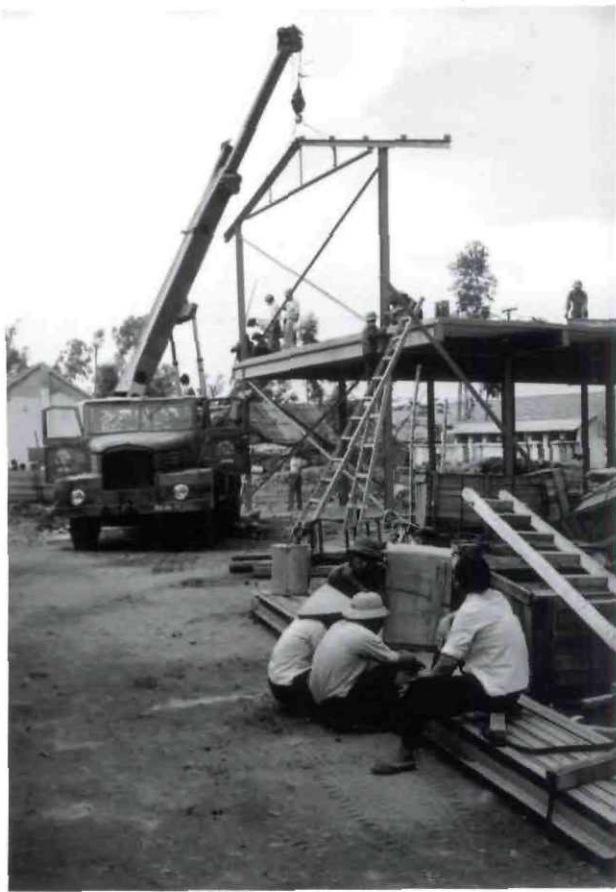
Above. The first frame on first floor was erected with the help of a crane. It could just as well have been done with a ginpole, but the lorry was at hand unloading door crates. In front engineers are discussing the designs.
